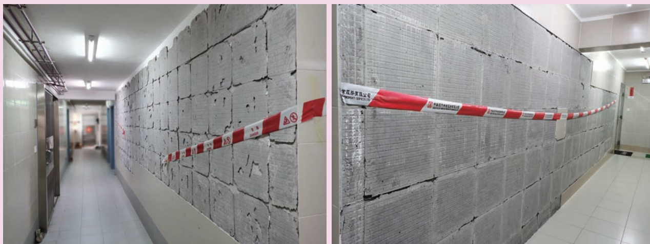
Large slabs of tiles have fallen off walls in the two economic housing projects including Edifício do Lago in Taipa and Edifício Ip Heng in Coloane
