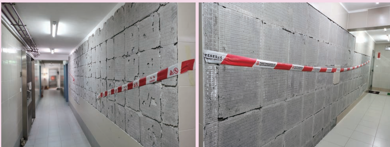
Large slabs of tiles have fallen off walls in the two economic housing projects including Edifício do Lago in Taipa and Edifício Ip Heng in Coloane
